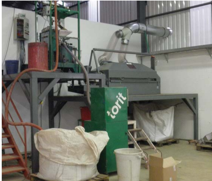
RFBD 600-12 connected to customer already in use coating system
