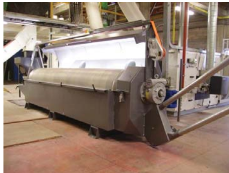
RFBD 600-19 Grass dryer connected to customer already in place coating system
